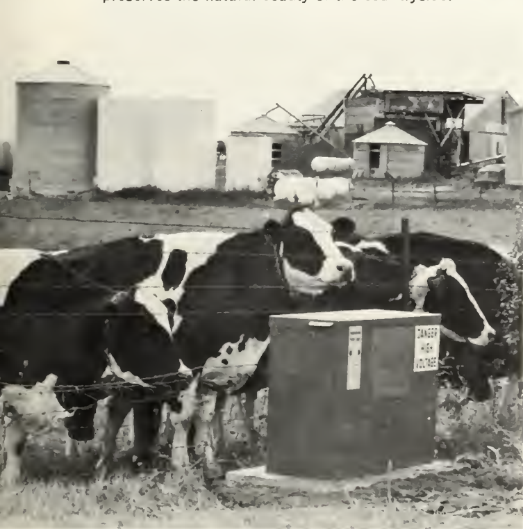
Once underground, little evidence remains of unsightly poles and wires. Hazards for people and livestock decrease.
